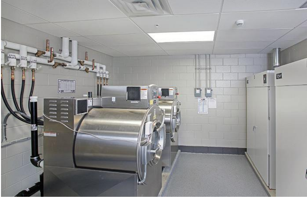
4 South River's fire headquarters station has two 105-pound-capacity washer/extractors that each can do six sets of turnout gear at a time and two dryers that each will handle six sets of turnouts.
