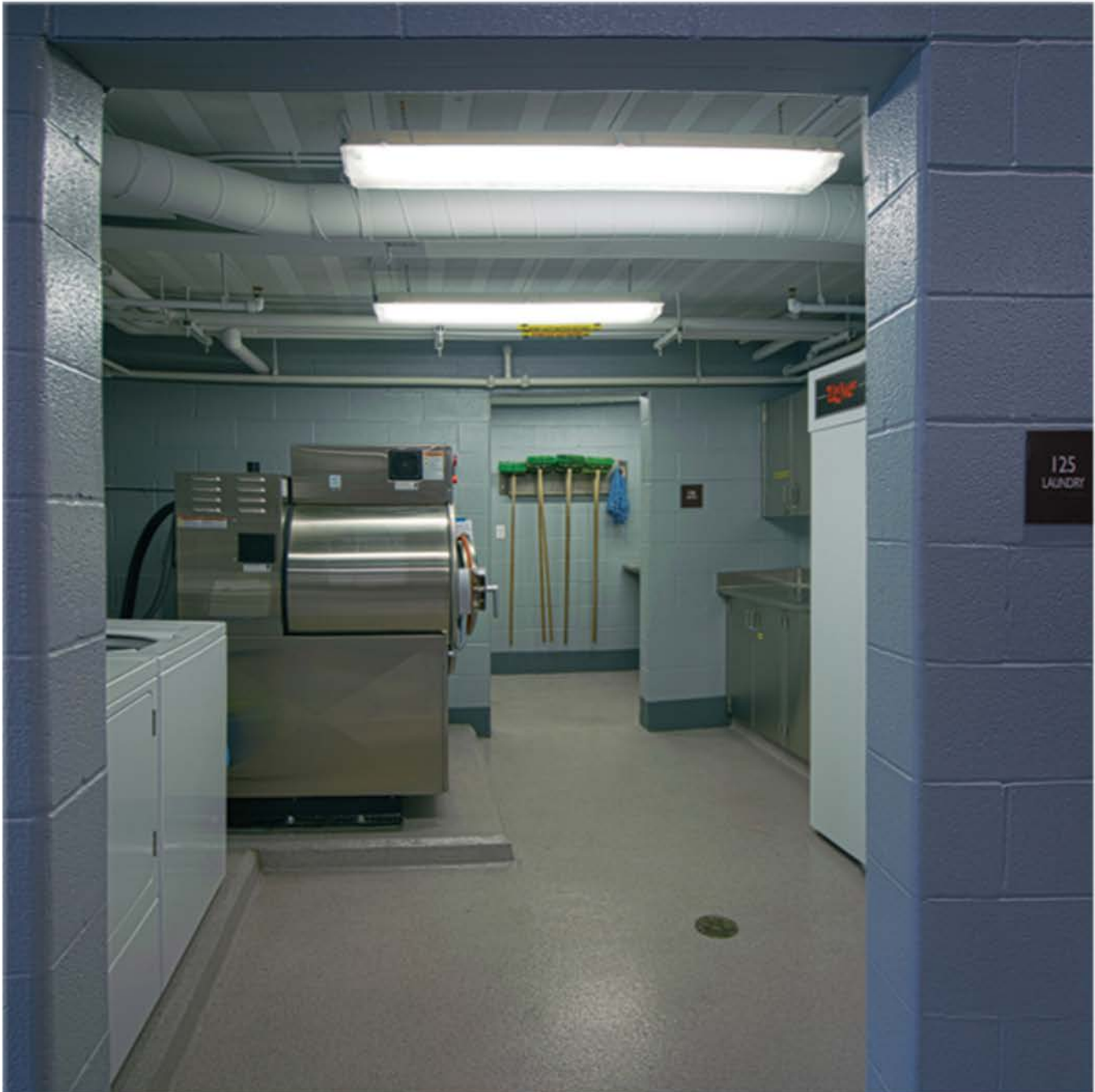
A decon laundry room is located on an outside wall adjacent to the apparatus bays.
